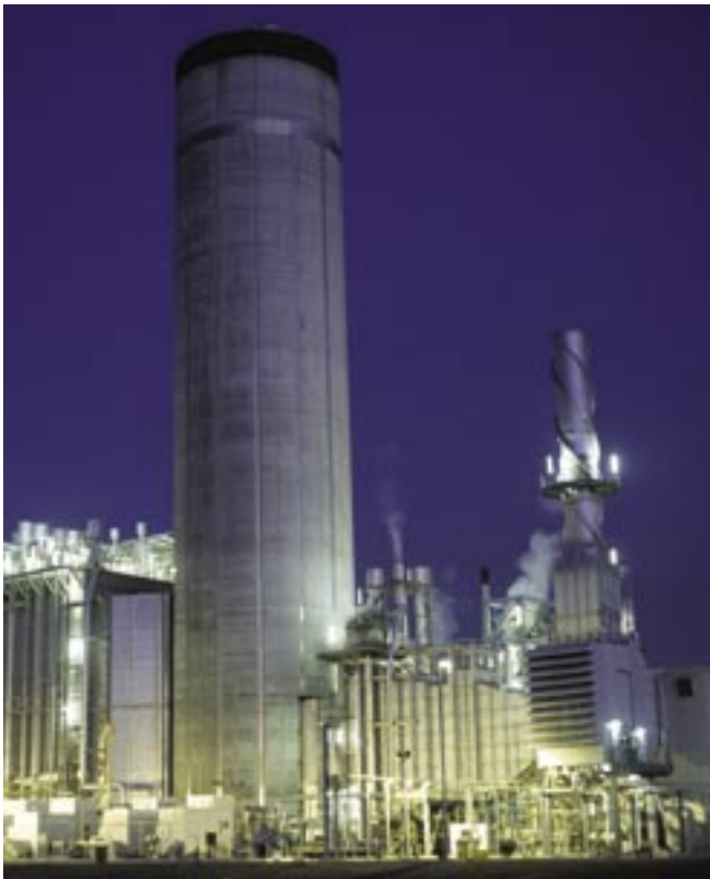
GE's H System is installed at the Baglan Bay Power Station in Wales.
