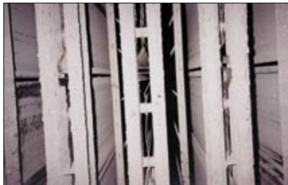
Fig. 6. Powerwave® acoustic horns cleaned the internal components of this precipitator so well, the plant stopped using the conventional tumbling hammer.
