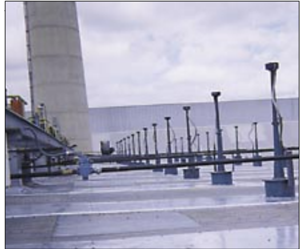
Fig. 8. Powerwave® acoustic horns mounted on the top of baghouse compartments.
