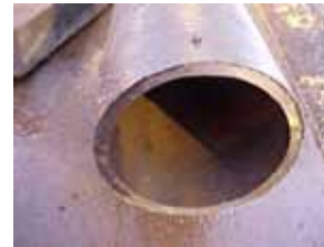
Cut section of casing
