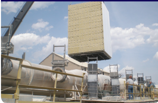
Figure 2: difficult crane access required 'flying' half of the compartments over the on-line system. Careful planning and close co-ordination were required to assure the compartment change-outs went smoothly
